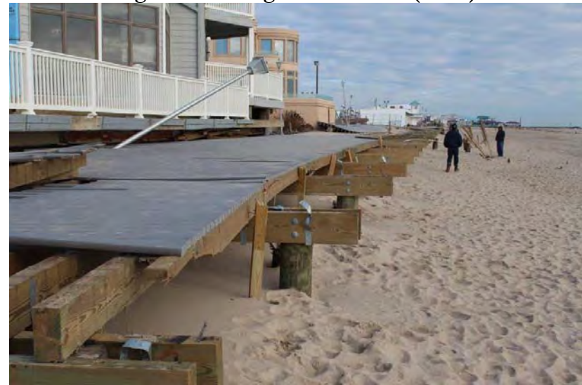
Figure 9: Damaged Boardwalk (1 of 2)
